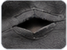
Open seam / broken seam
